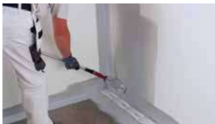
Apply first coat of LIP VS30 to all areas shown below using a roller.
