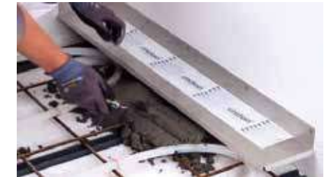
Pack the outlet and underside of the drain with screed making sure there are no air pockets.
